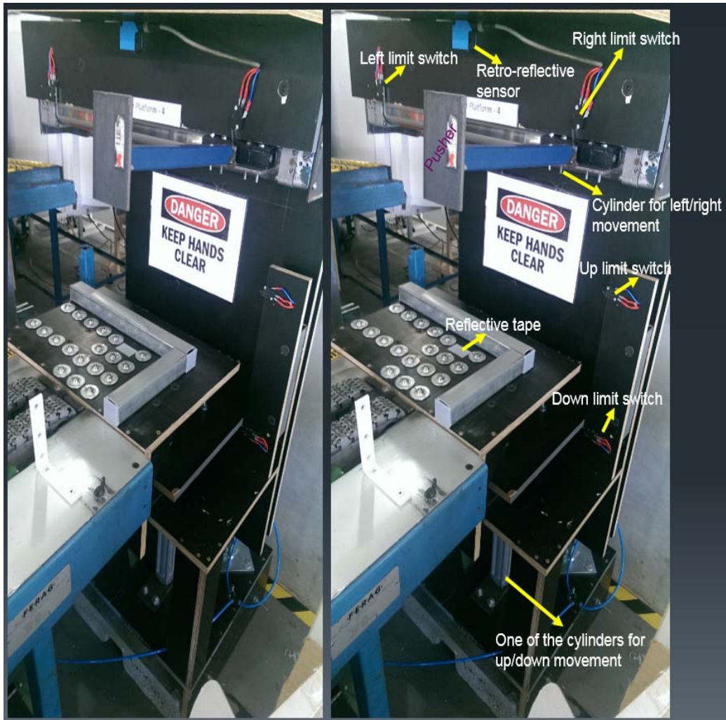
Figure 28: Front view of transfer platform 4
