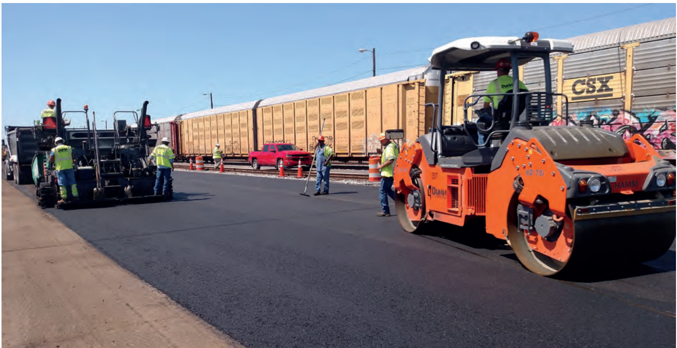
A railway freight yard, such as the CSX Total Distribution Services Inc. (TDSI) facility in Birmingham, Alabama, is typical example of an area that requires a heavy-duty pavement. (Photo courtesy Dunn Construction)
