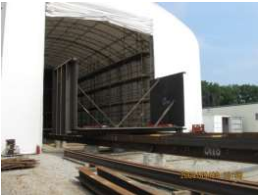
Figure 1-This photo shows the C Section of duct going into the tent.
