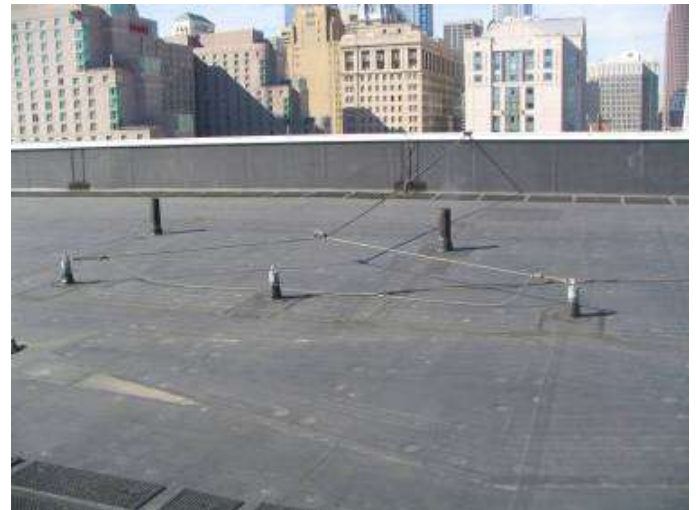
This photo shows permanent roof anchors. Specifying multiple roof anchors will provide convenient tie off points when working near the edge of the roof.
