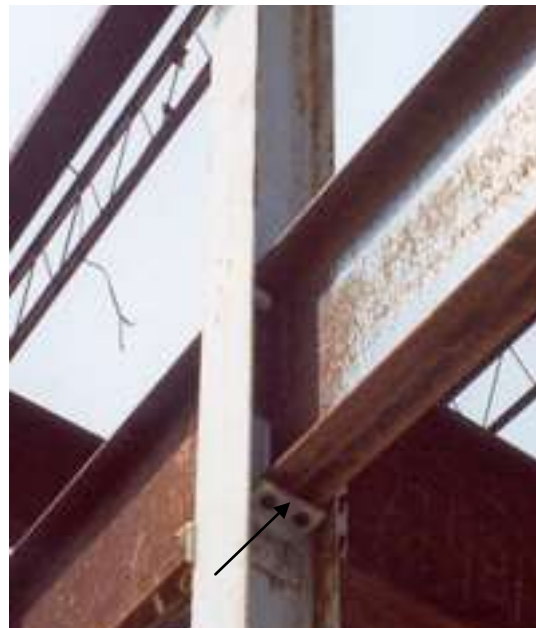
Design safety seats (see arrow) at column connections. The safety seats eliminate hanging connections making the connection process easier.
