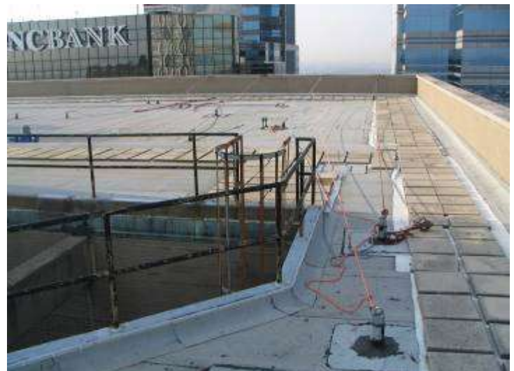
This photo shows guardrails installed along an opening. Installing guardrails early on in the construction process can eliminate the risk of a fall through an opening.
