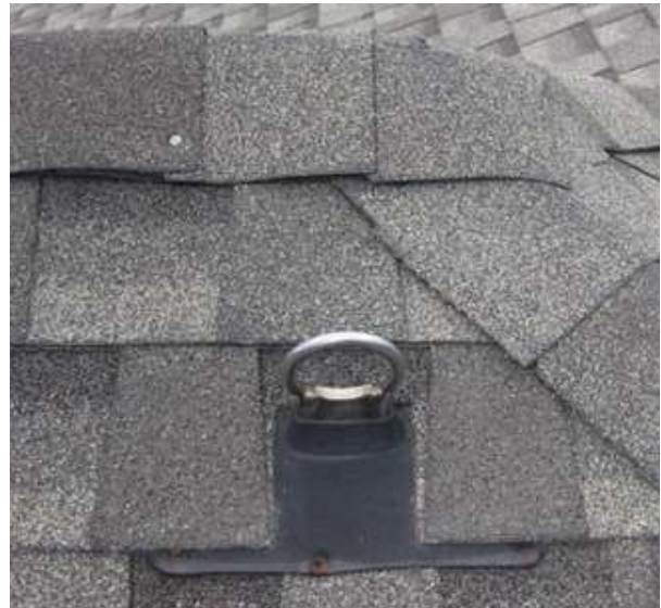
Figure 2 Residential roofing has a high incidence of falls. Residential roof anchors properly installed provides a place for workers to anchor to during future maintenance.
