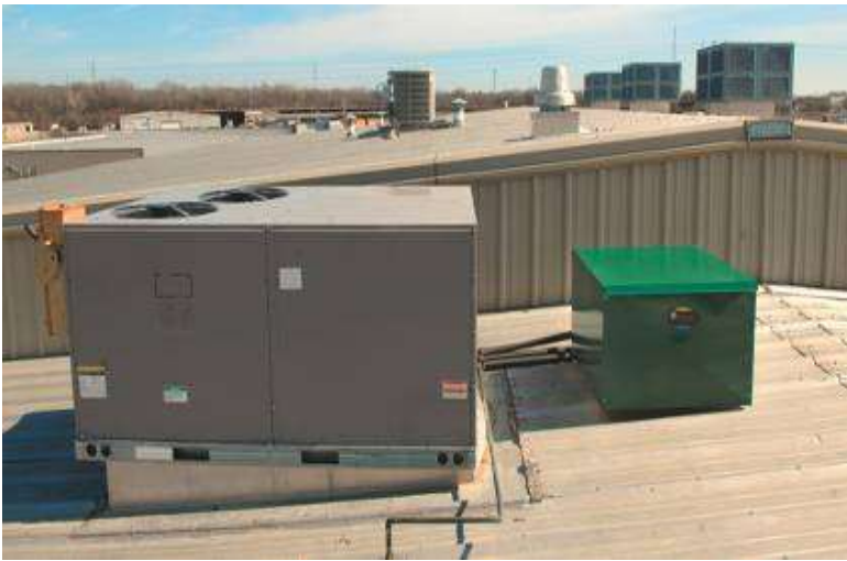
This photo shows equipment located on a roof. Positioning equipment at least 15 feet back from the roof edge will reduce the risk of falling when installing and servicing the equipment
