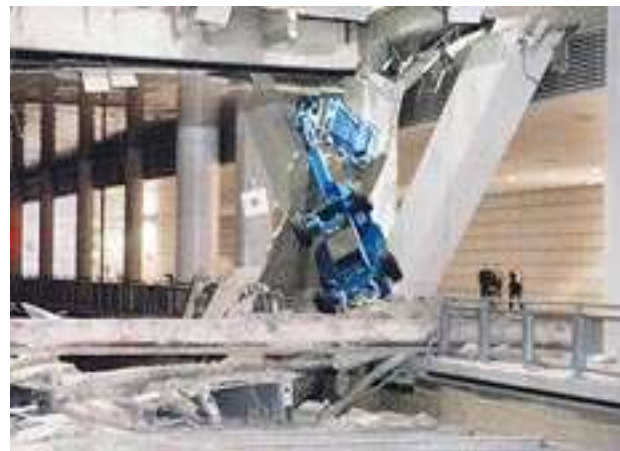
Figure 2 Structural collapse from weight of equipment
