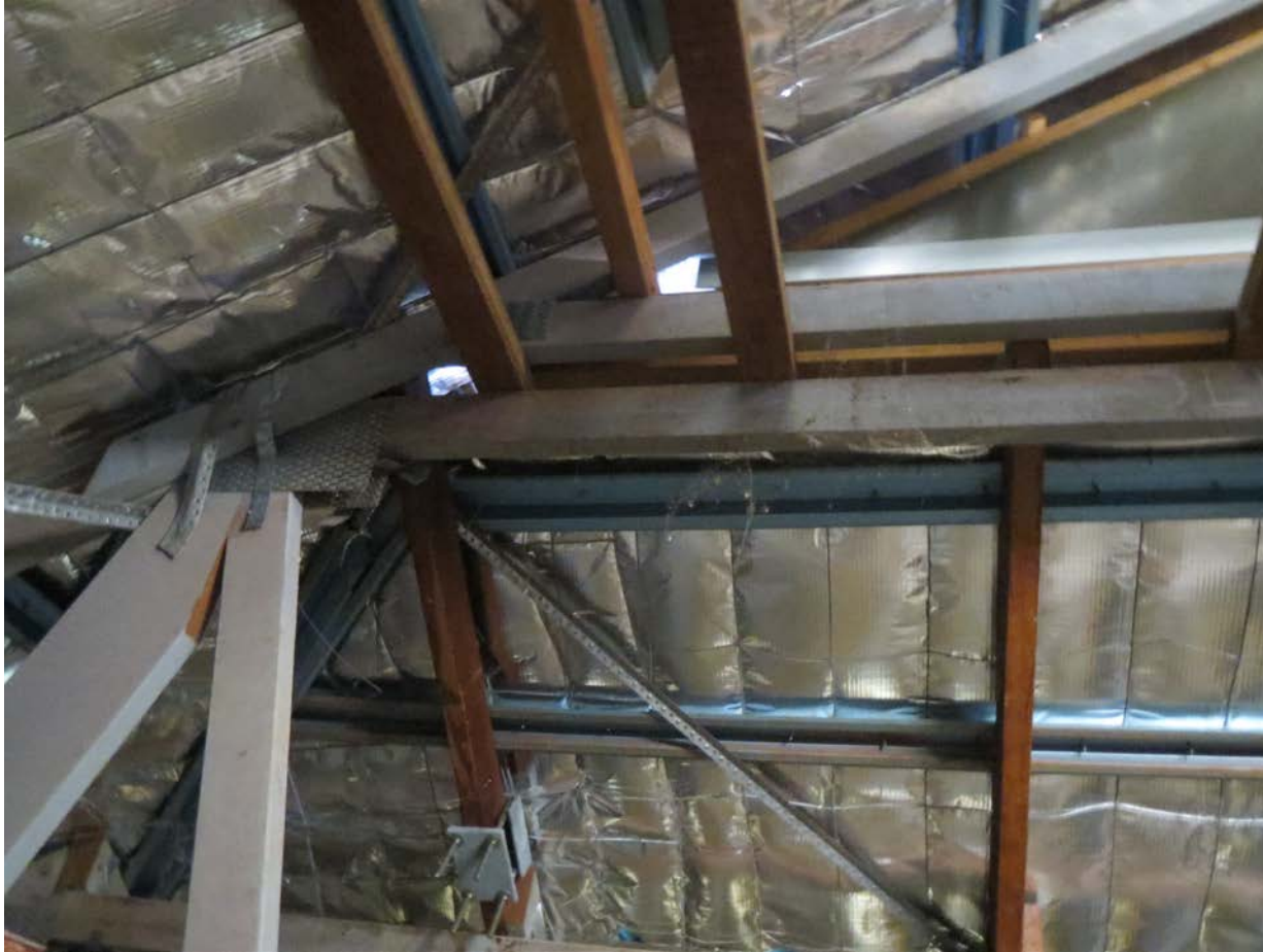
Failure of vapour barrier
