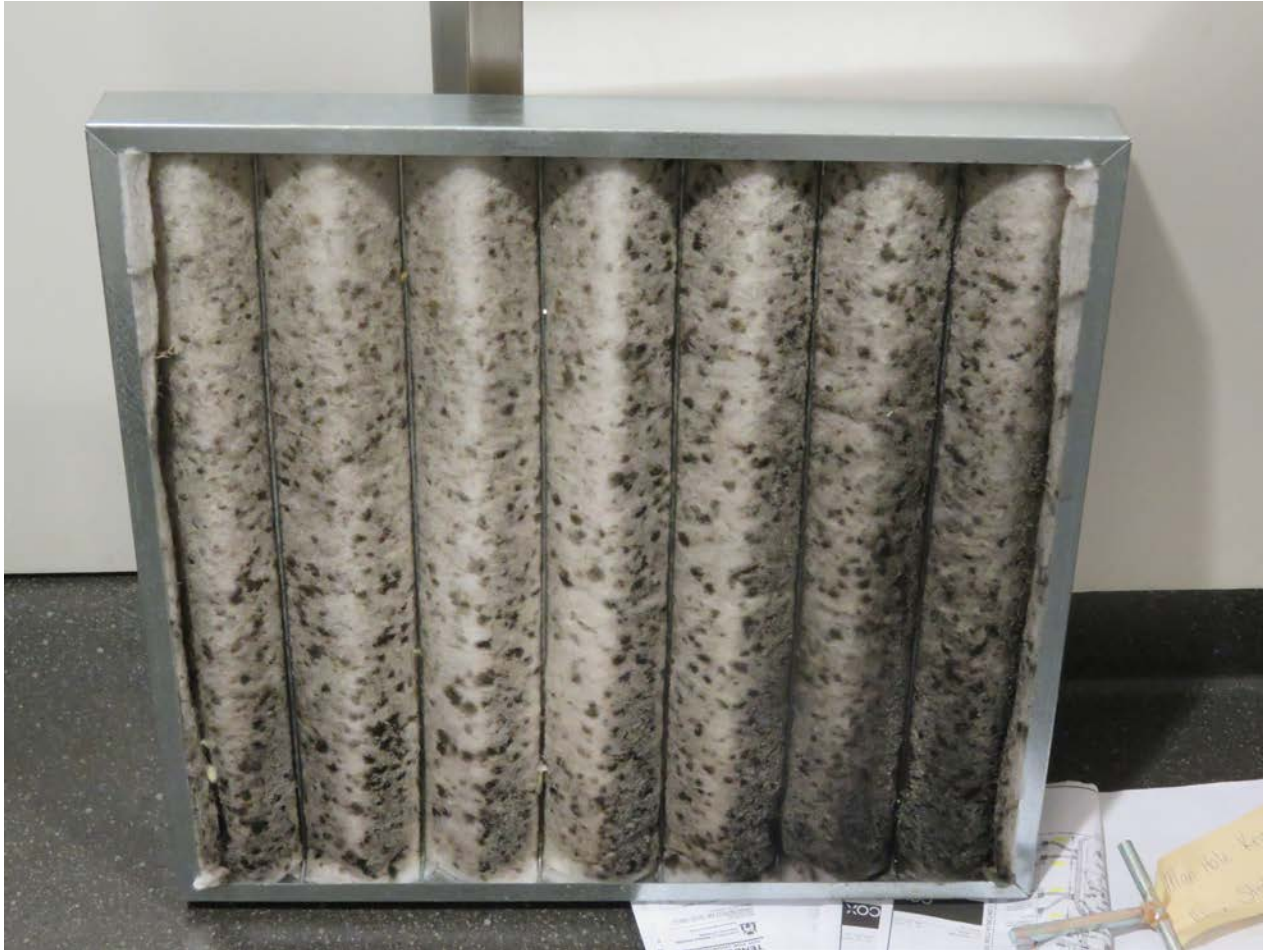
Carnarvon – saturated return air filter from secondary FCU
