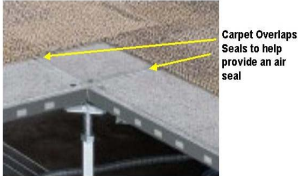
Figure 15 – Carpet used to prevent plenum leakage
