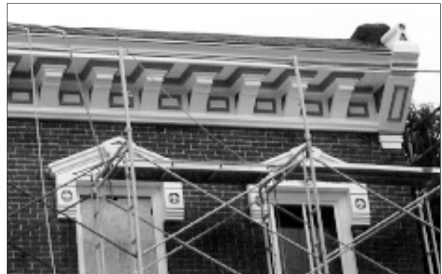
Repair only those features that are deteriorated. Above photo is the "before" condition of the lower image. (St. Charles, MO)
