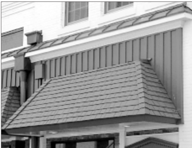
Odd shaped awnings are inappropriate on most historic structures.
