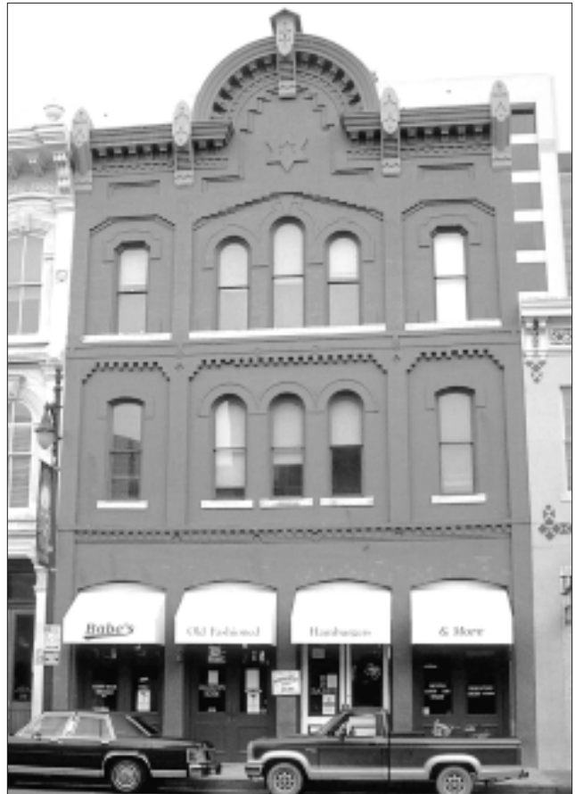
If a storefront is covered or obscured with a later alteration (top photo), then restore the storefront to its historic character. (Austin, TX)
