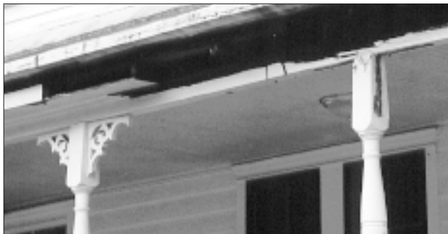
Replace missing original details in kind.
