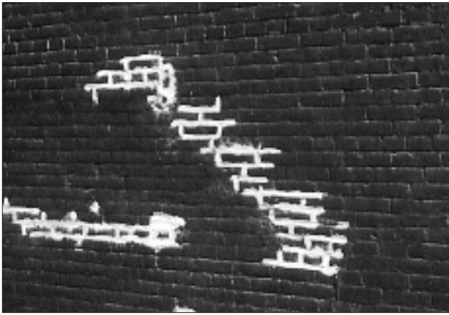
Avoid using mortar with a high portland cement content, which will be substantially harder than the brick and does not allow for expanding and contracting. The result is deterioration of the brick itself.
