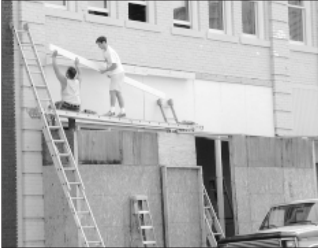
Replace missing original details in kind. (Greenville, SC)
