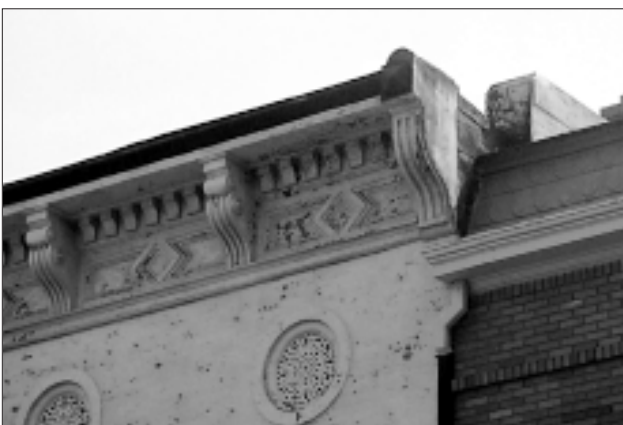
Many cornices are made of sheet metal. Areas that have rusted through can be patched with pieces of new metal.
