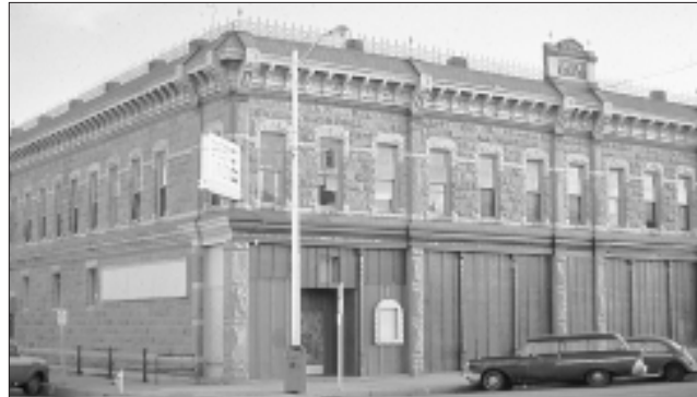
The windows in this structure were boarded and architectural details needed repair. (Compare with the photo below.)
