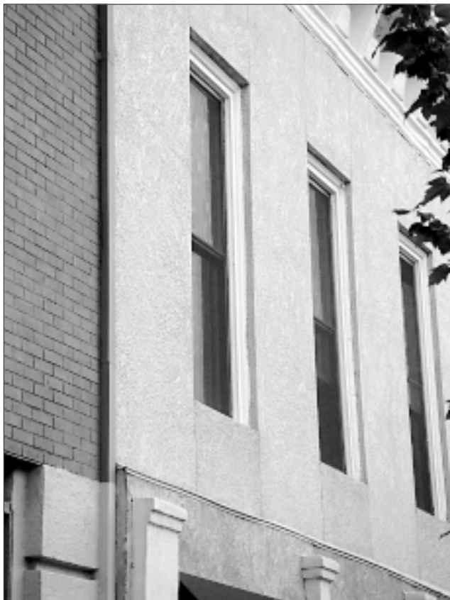
Covering the original building materials is inappropriate.
