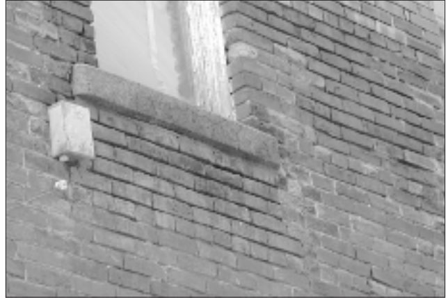
Protect masonry from water deterioration.
