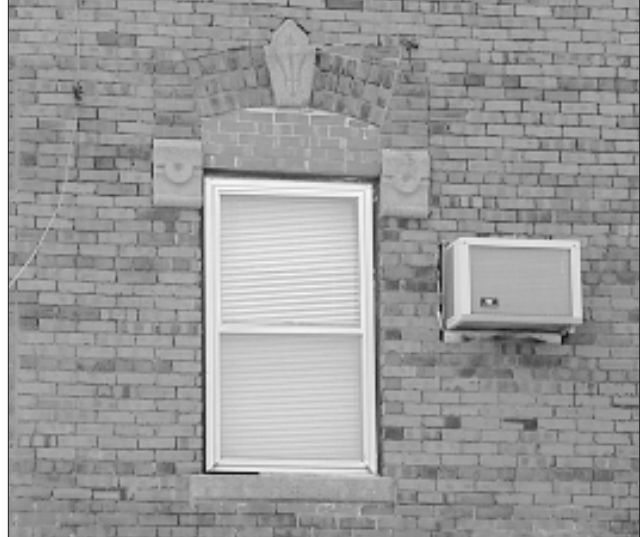
Do not locate window air conditioning units on a building's primary facade.
