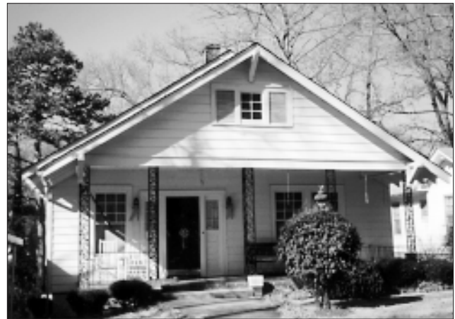
This porch has experienced an inappropriate alteration; wrought iron supports have replaced wood piers. Compare it with its "twin" in the photo below. (Spartanburg, SC)
