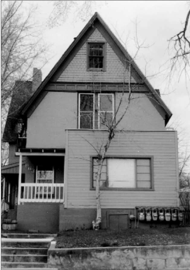
Design a new addition such that the original character can be clearly seen. This addition to the front of the historic structure is inappropriate.
