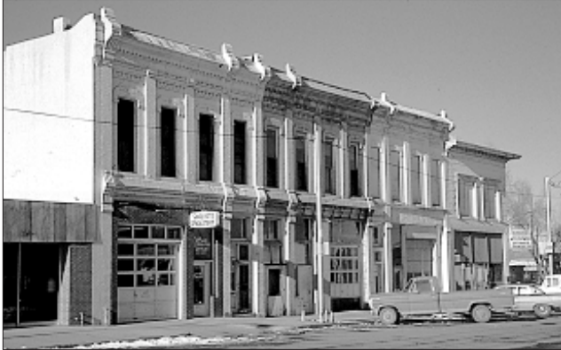
This row of buildings had lost some details over time and a monochromatic color scheme obscures the original design character. Overhead garage doors that had replaced original storefronts were later alterations without historic significance. (Compare with the “after” photograph below.)
