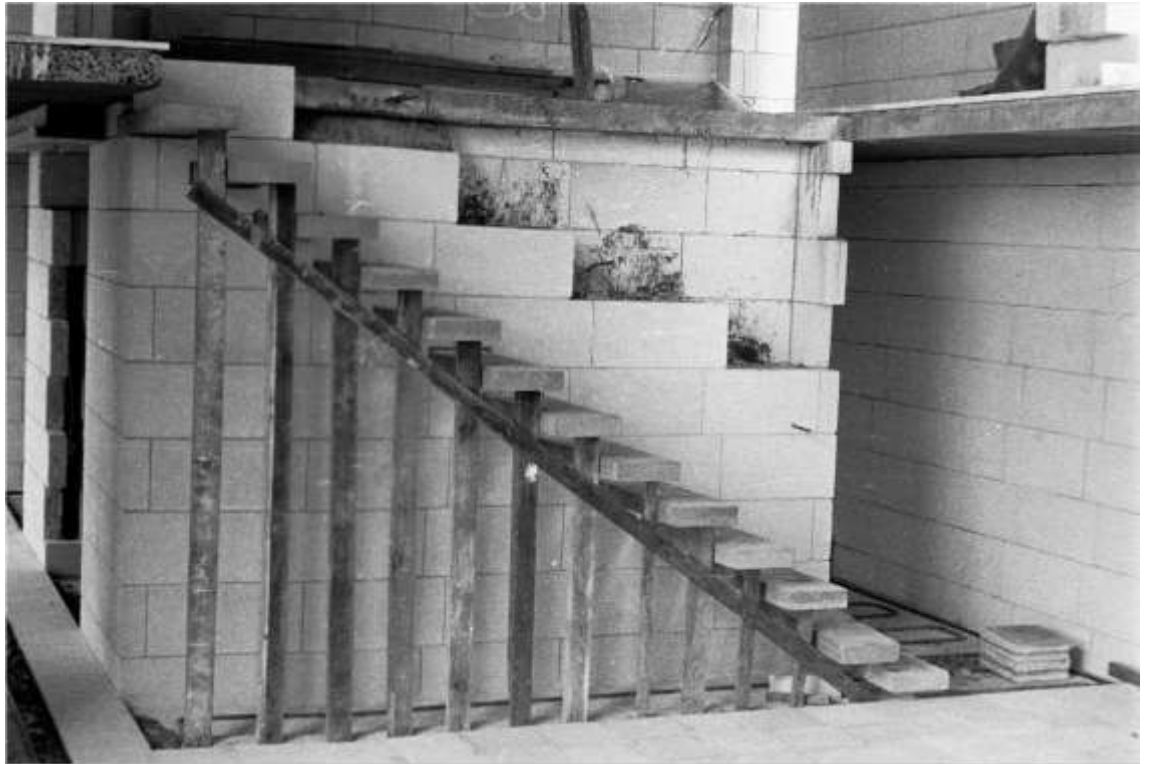
Reed house (Heide II) 1967 living room, cantilevered staircase under construction Photographer unknown State Library of Victoria, Barrett Reid papers, MS 14854
