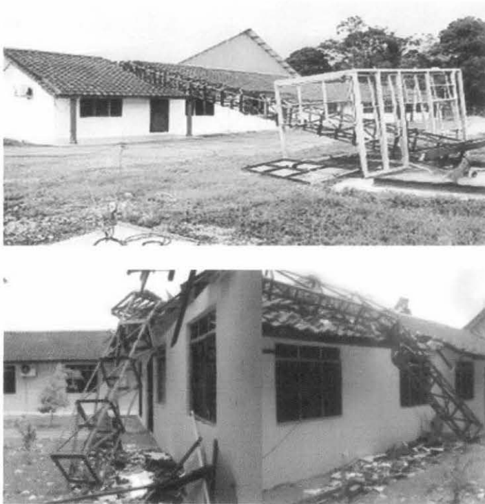
Figure 5. Menara Mobile Mast Found Collapsed on August 1 st 2009.
