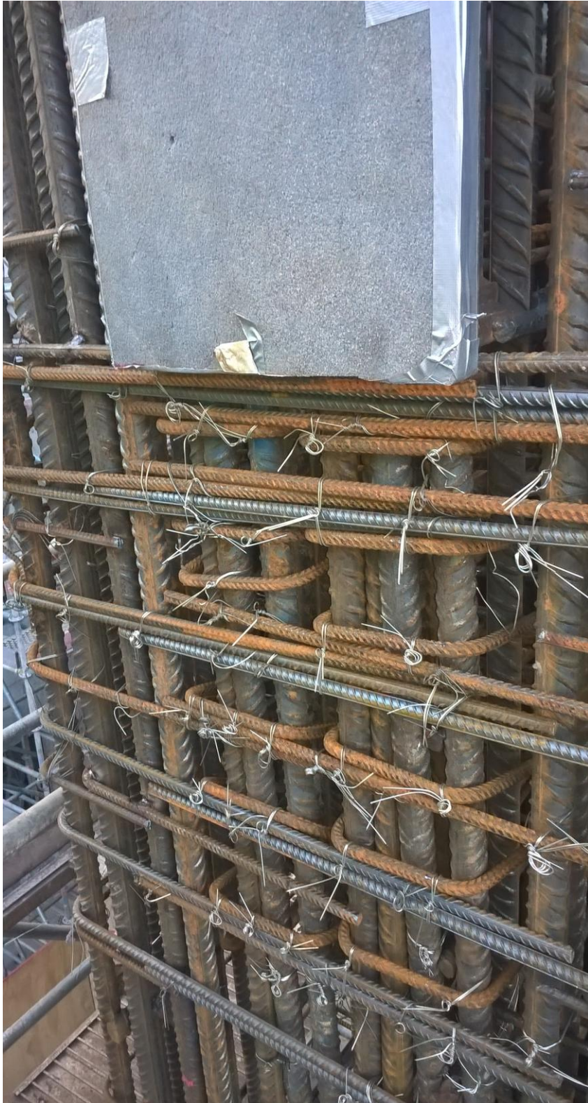
Figure 2. Too densely reinforced concrete structure. (Sweco Rakennetekniikka Oy. 2017)
