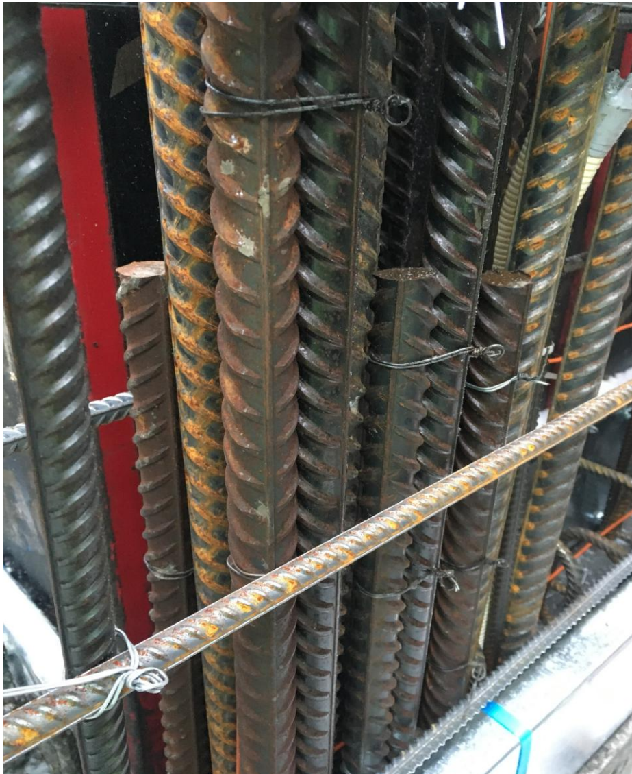
Figure 1. A row of rebars installed for a wall at construction site. Too little space is left for vibration work.
