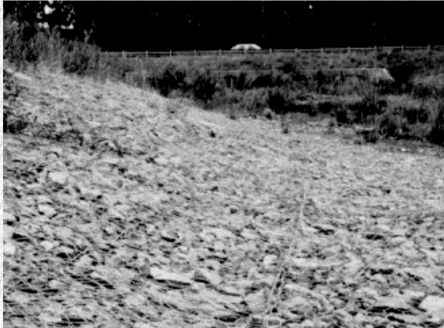
Figure 9. Rock and Wire Mattress Revetment
