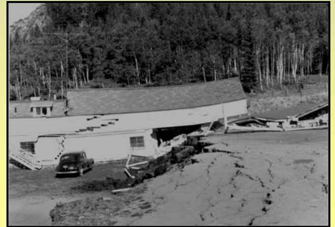
Photo; USGS- Damaged and collapsed buildings at the Blarneystone Ranch, near Hebgen Lake, Montana, caused by the August 18, 1959, earthquake. (Photograph by I.J. Witkind.)
