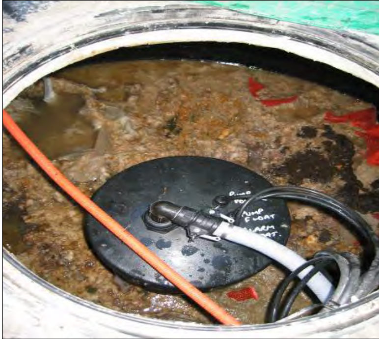
Figure 5.10 A flooded system due to pump failure
