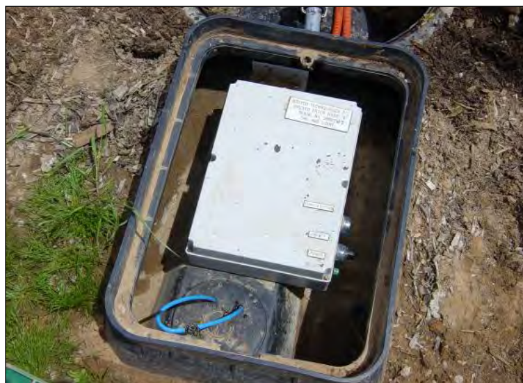
Figure 5.8 An electrical box that was flooded
