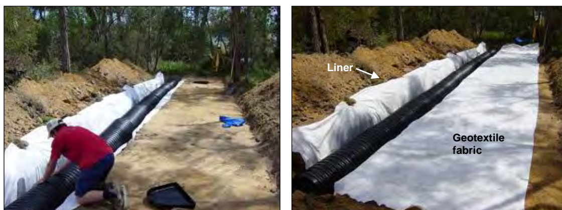
Figure 10.16 and 10.17 Laying the liner in the trench and then the geotextile fabric as the 'wick' across the pan
