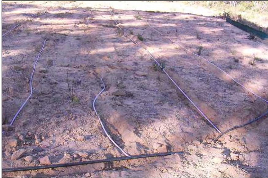
Figure 13.7 Poorly installed subsurface effluent irrigation system
