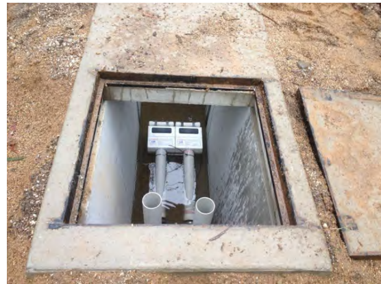
Figure 10.4 Flout in dosing chamber
