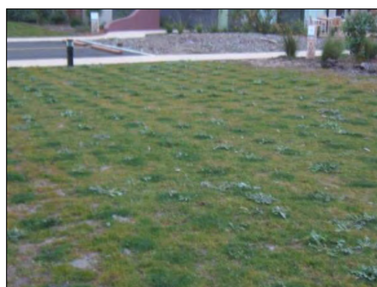
Figure 13.2 An installed subsurface irrigation system with close emitter spacing (Whitehead & Associates)
