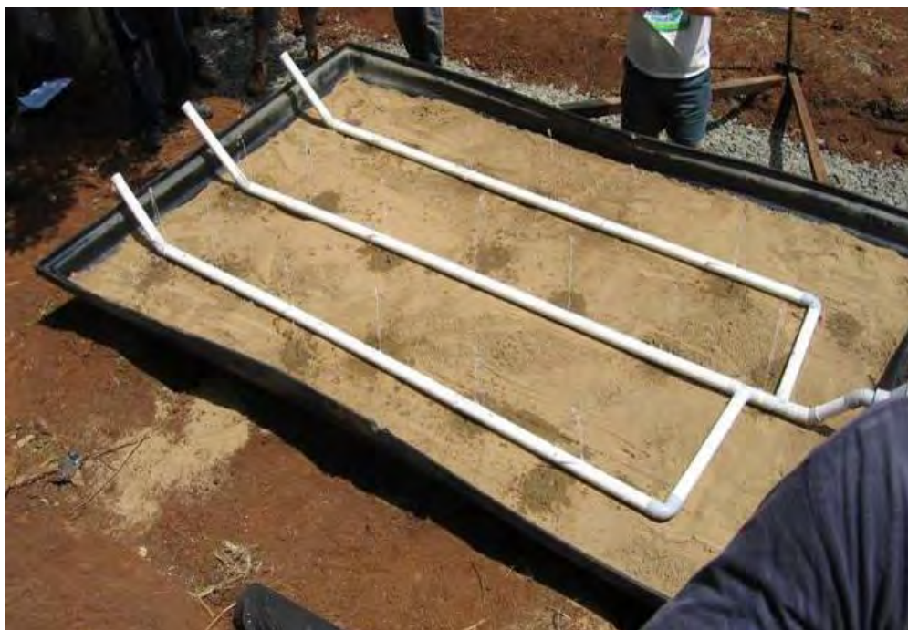
Figure 14.3 Siphon being tested delivering pressure dosed load to a sand filter (Whitehead & Associates)
