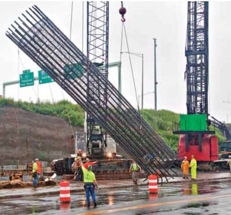
Fig. 7: A well-braced drilled shaft cage is picked with minimal distortion (photo courtesy of Dimension Fabricators, Inc.)
