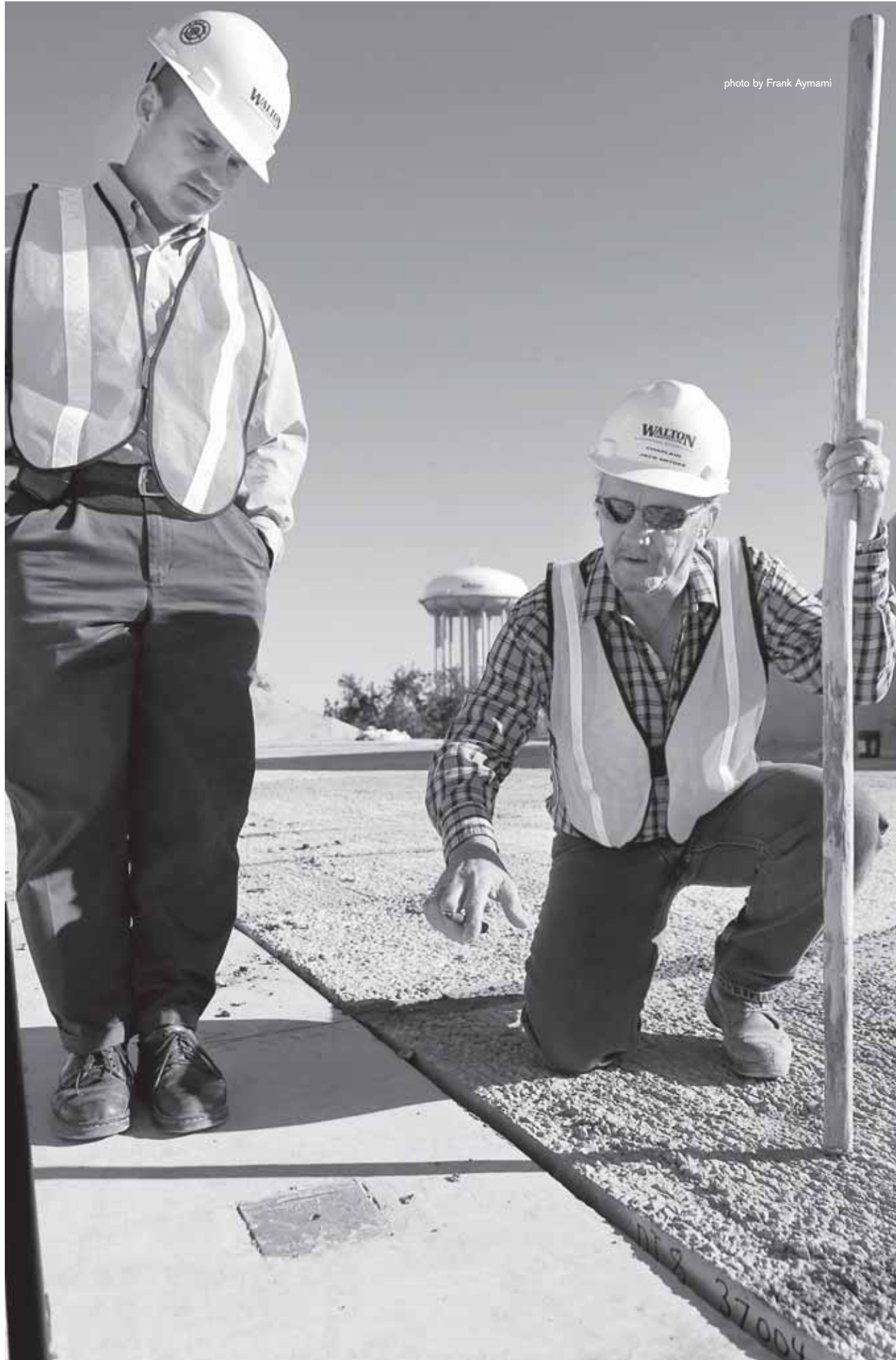
Walton Construction employees Jeff Mobley, left, and Jack Snyder review roof details at a Jackson Barracks project.
