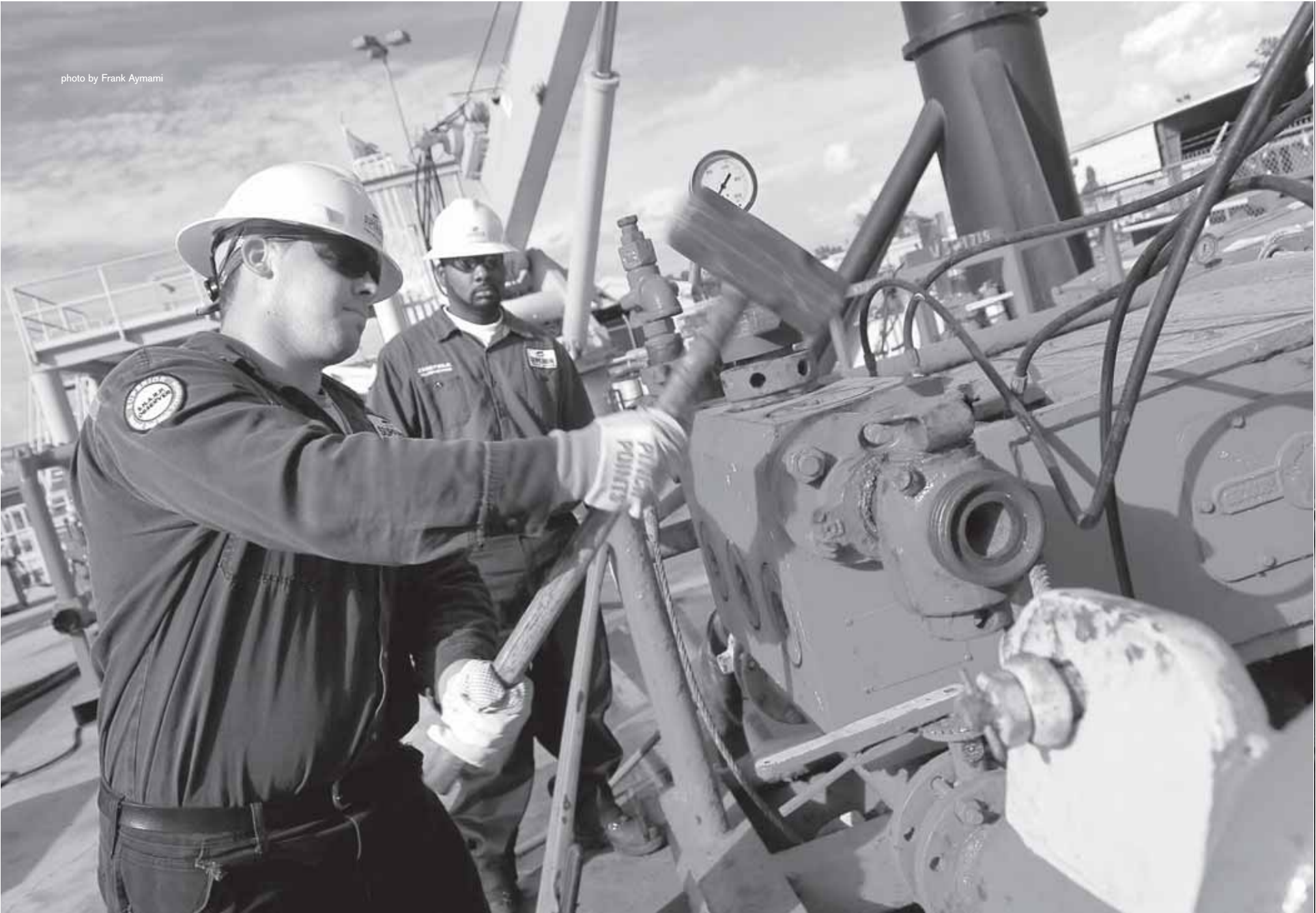
Pump operator Tim Miller, left, and crane operator Jerome Fobb Jr. prepare a pump at Superior Energy Services' Harvey facility.
