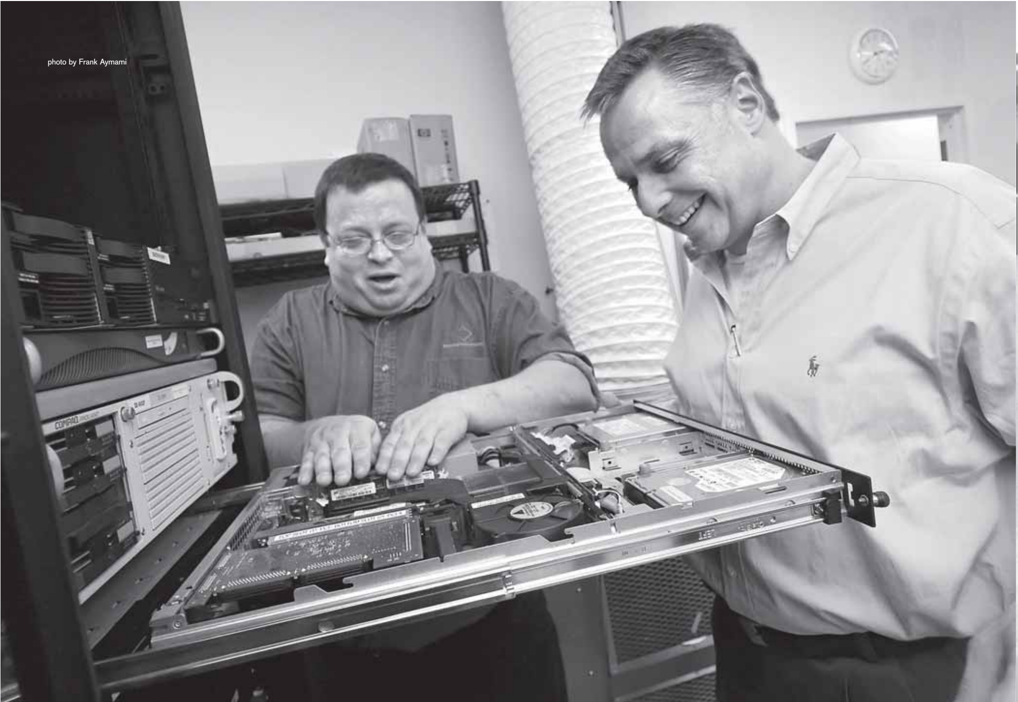
Network engineer Robert Breland, left, and CEO Joey Auer work in Diamond Data Systems' server room.
