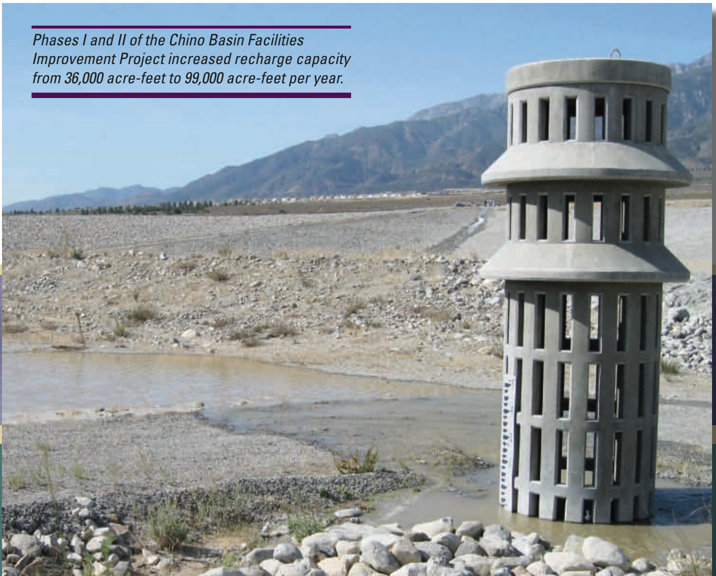
Riser outlet tower at the Etiwanda Debris Basin.
