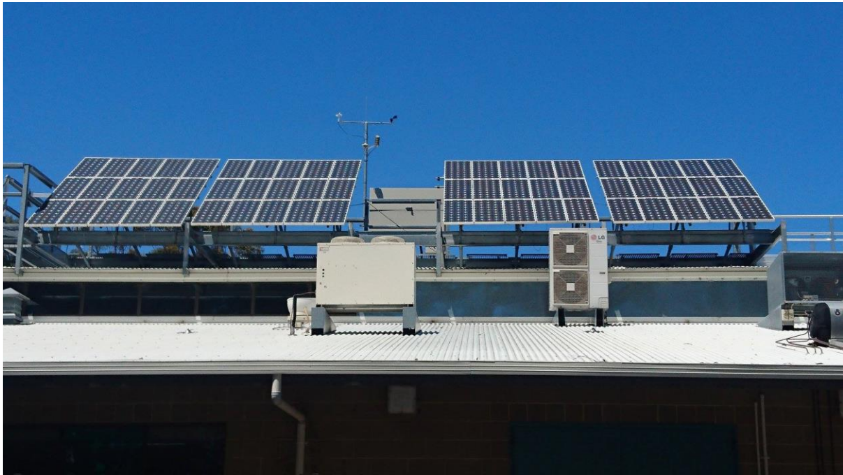
Figure 3: PV Array on Building 190 Rooftop
