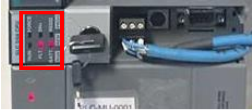
Figure 24: Initial PLC Fault Conditions
