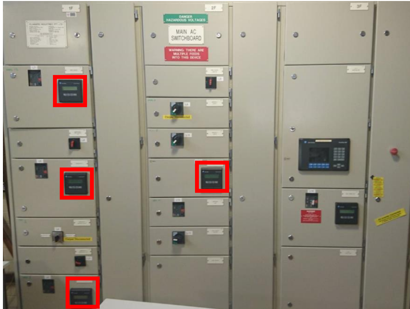
Figure 37: Powermonitors That Have Been Disconnected
