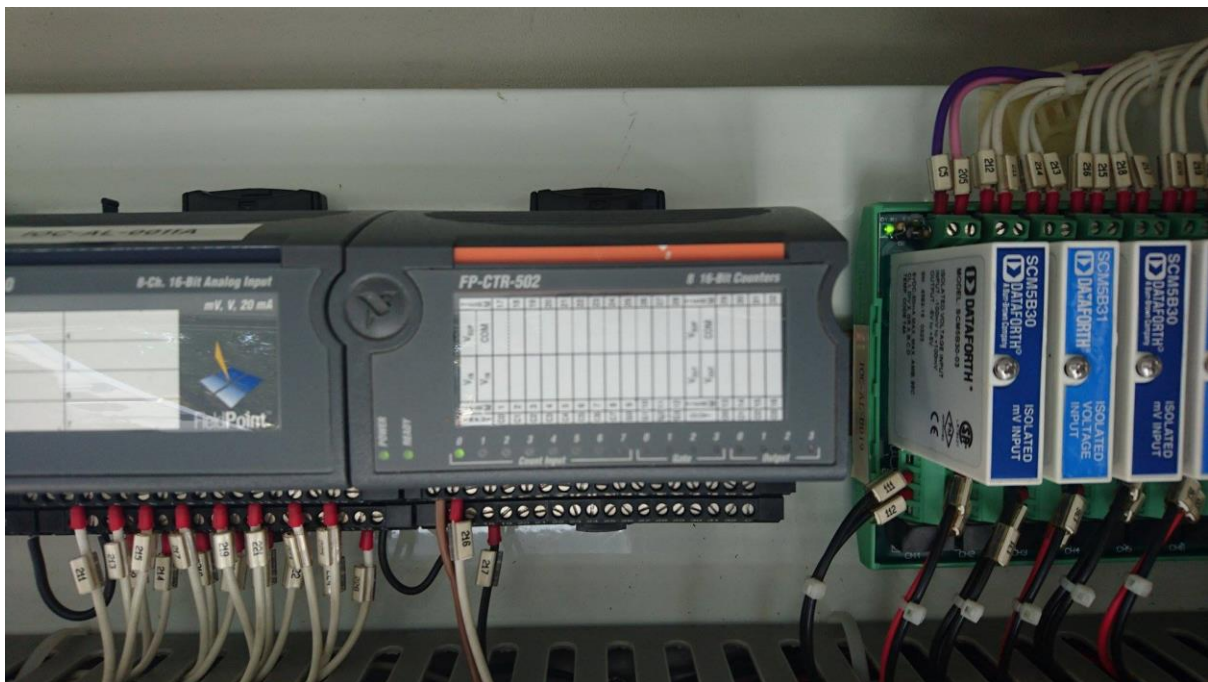
Figure 11: FP-CTR-502 Module Installed in Patch Panel
