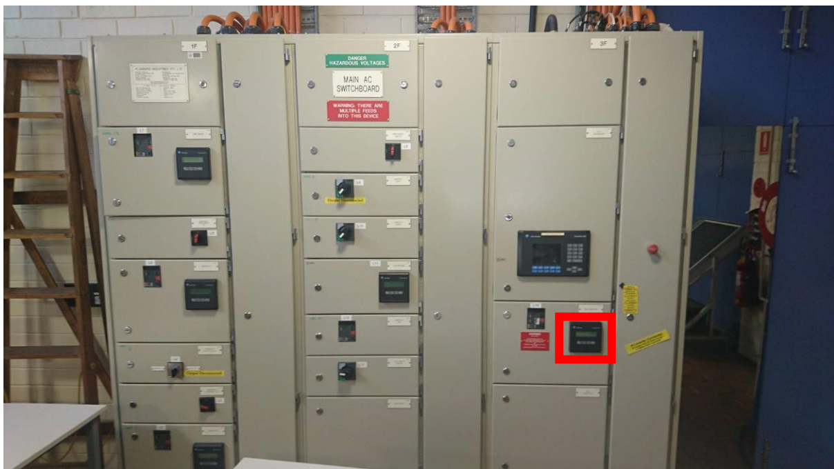
Figure 31: Powermonitor Responsible for Measuring Power Delivered to Grid in MACSB
