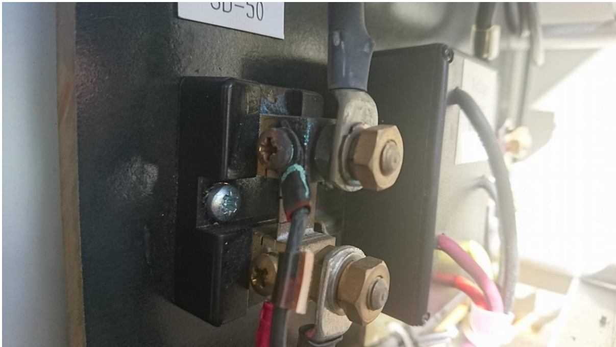
Figure 22: Blackened 50A/50mV current shunt on Block D
