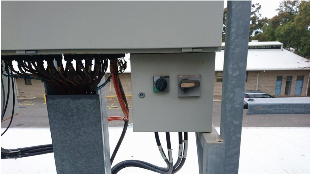
Figure 36: Rooftop Switches Prone to Tripping
