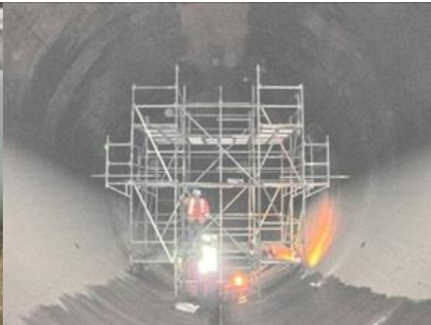
Figure 7: Internally Mounted ATF
