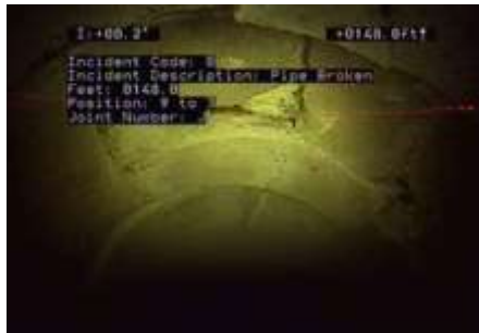
Figure 7-4: Broken Pipe Due to External Loading
