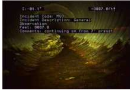
Figure 7-3: Sediments and Corroded Pipe
