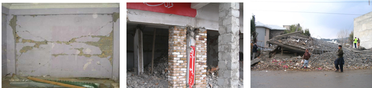
Fig. 2: Observed damage states of RC buildings during 2005 Kashmir earthquake: shear cracks in masonry infill, moderately damaged building (left) [11], heavily damaged and collapsed infill with significantly damaged RC columns, extensively damaged building (middle) and collapsed building (right) [3].
