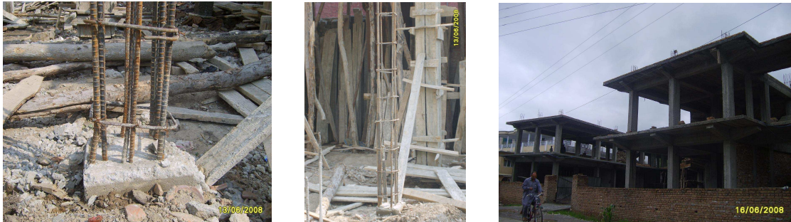
Fig. 1: Column reinforcement and detailing, column-to-foundation connection (left), spacing of transverse reinforcement (middle), lap-splice provisioned for floor-to-column connectivity (right), observed in the valley of Abbottabad.
