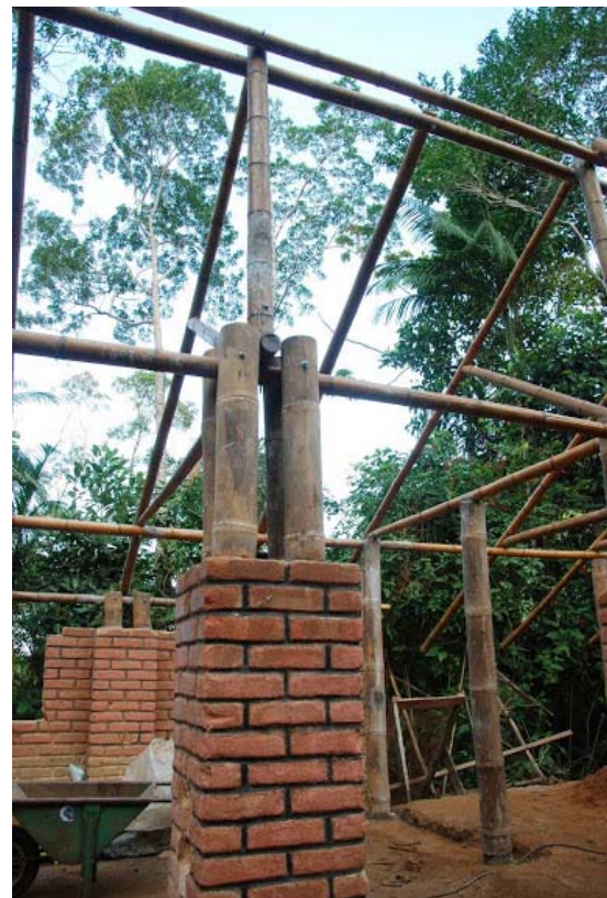
b) Construction of welcome center with overbuilt columns supporting simple roof structure.
