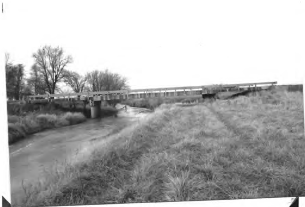
Figure 16. County Road 300 North multi-span bridge over the Embarras River near Pesotum, Ill.
