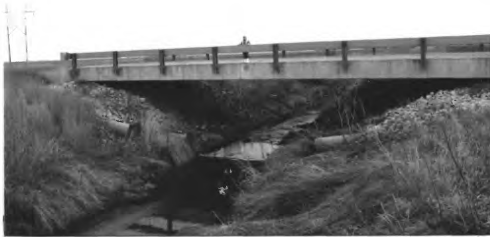
Figure 14. County Road 2050 East single-span bridge over Flatville Drainage Ditch near Flatville, Ill.
