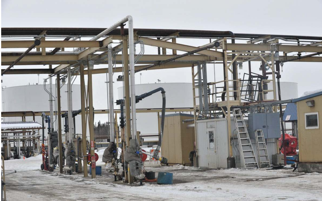
Figure 9. Diesel fuel delivery station at PetroStar Refinery, North Pole, Alaska. The gray building just to the right of center houses the metering and injection of additives. Truckers enter orders for fuel and fuel blends in the brown building at the front right of the gray building. They use an advanced control and metering system for dispensing the requested fuel into delivery trucks positioned in the station. Fuel storage tanks can be seen in the background. Photo by Frank Williams.
