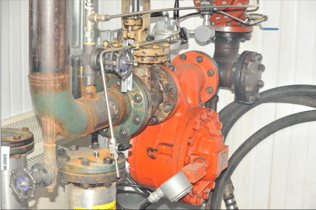
Figure 11. Mixing point for lubricity additive. Lubricity additive enters the fuel stream from the electronic metering system through the smaller gray isolation valve left of center above the large green elbow. The additive mixes with fuel flowing in the larger pipe with a green elbow. The fuel and the additive mixing is assured as the components flow through the meter (orange) and on to the awaiting truck. Photo by Frank Williams.
