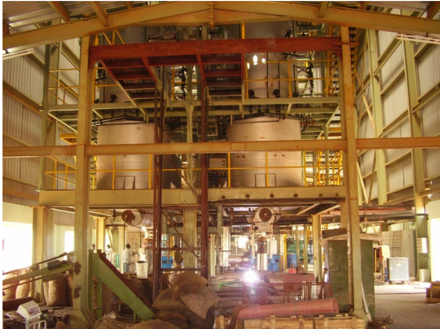
BMC GASIFIER PLANT(1700Kgph)
