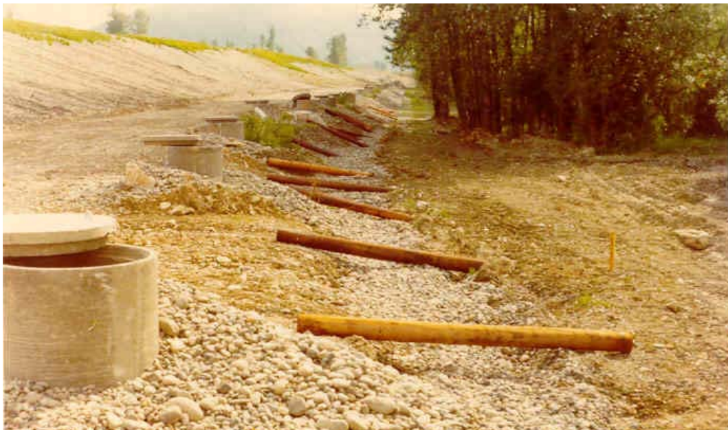
Photograph 9: Pressure Relief Wells
