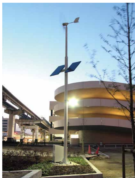
Osaka Airport, Japan wind & solar hybrid lighting system in 2004
