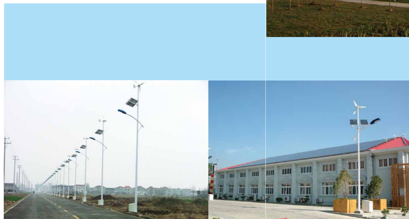
Shanghai Chongming island wind & solar hybrid lighting system in 2004
