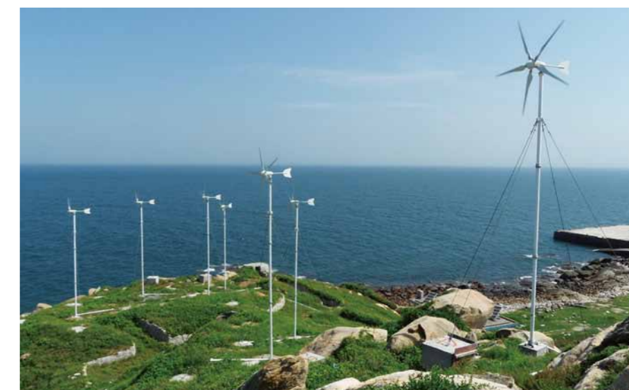
Nanpeng Island wind & solar powered seawater desalination system in 2010
