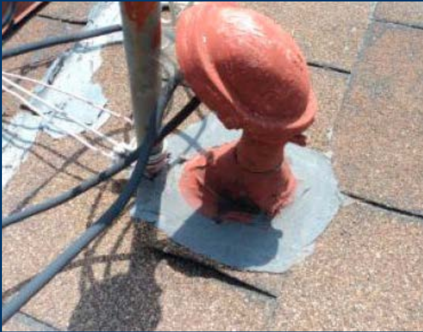
Electrical service drop on roof
