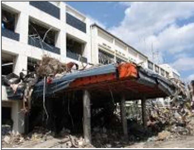
City hall at Rikuzentakata in Iwate Prefecture
