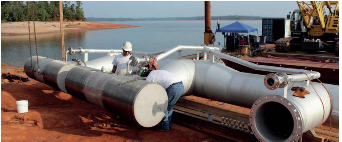
Johnson Screens® Passive Intake Installation: Drinking Water Plant, in South Carolina, USA
