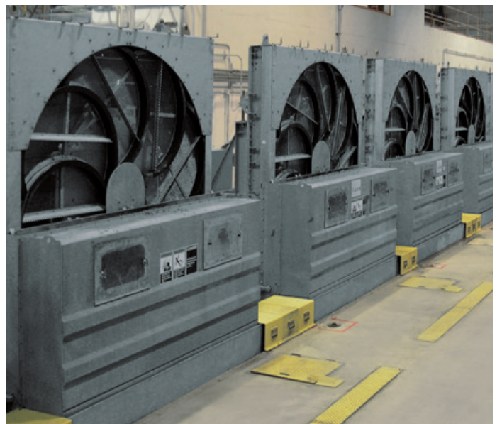
DC Cook Nuclear Power Plant, USA
