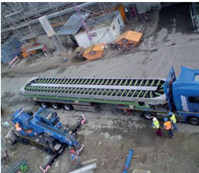
GKM 9 Power Plant, Mannheim, Germany
