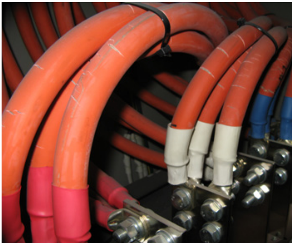
Unsafe: An installation of Deltaflex electric cable with clearly visible cracks in the protective sheath that pose a risk of electric shock or fire.
