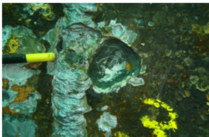
Figure 3-1 An example of outboard splash zone is shown in the photograph, showing pitting on the plating and weld cap. The pit was found to be 10 mm deep and 50 mm in diameter.
