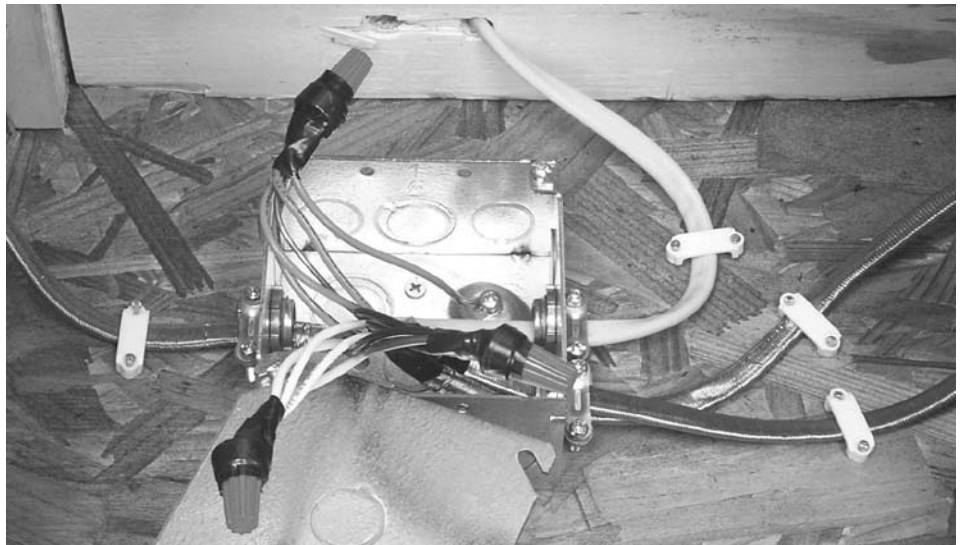
Junction box with multiple sets of mat lead wires, connected in parallel, and connected to the SunStat control above.
