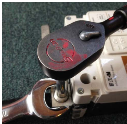
Figure 4.7 – Lug Damage Prevention
