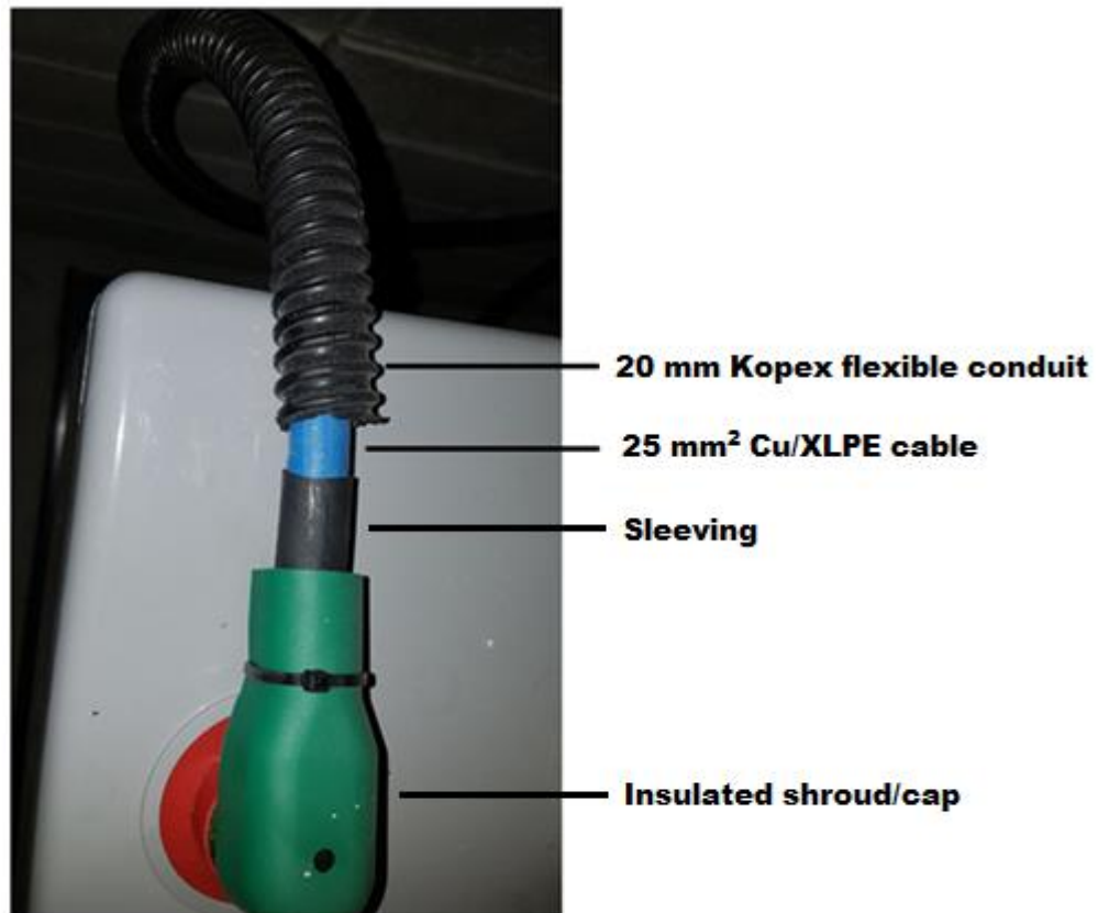
Figure 4 - Close up of Battery Termination
