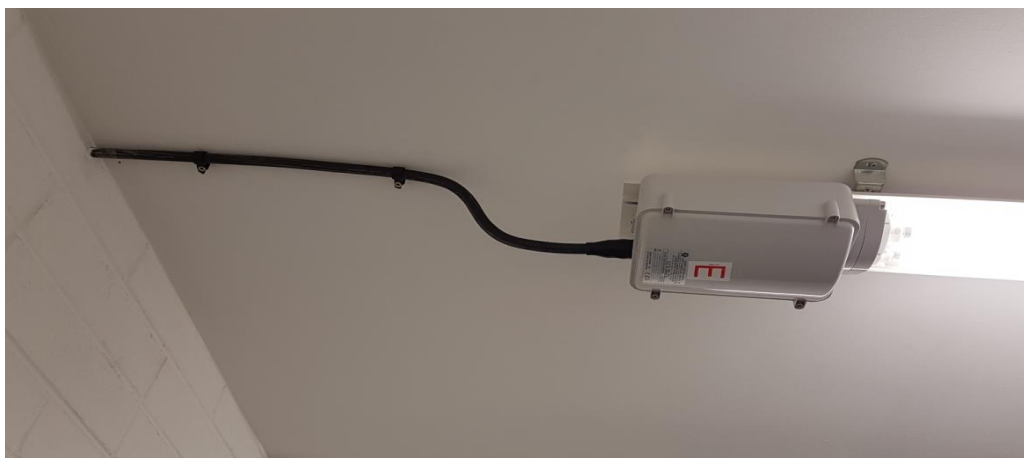
Figure 5 - Example cable wiring to Ex light fitting
