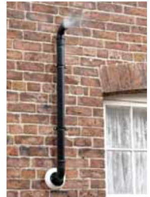
Installed to prevent nuisance plumbing across the window
