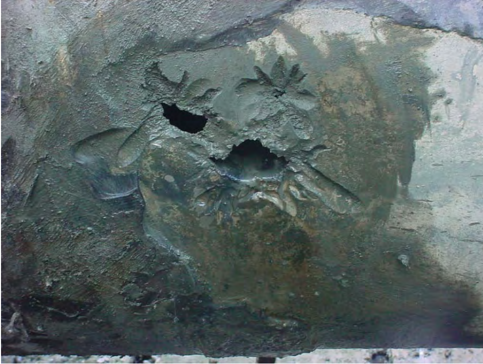
Figure 1 Photo of leak at MP 28.
