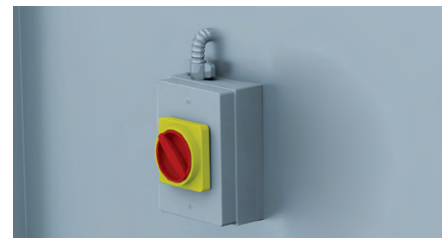
NEMA 4 Disconnect Switch
