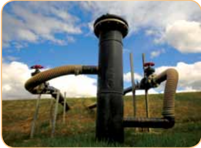
An extraction well collects gas from the landfill and routes it to the new landfill gas-to-energy facility for conversion to marketable natural gas
