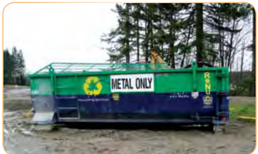
Separation of materials with economic value, such as metals, at a construction site can help reduce project costs.
