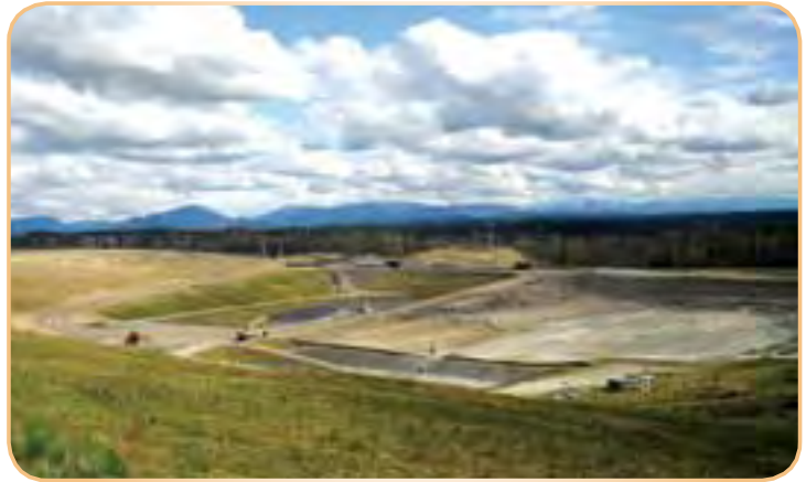
The landfill has been developed in sequential stages (or refuse areas), with construction of Area 7 currently in progress.
