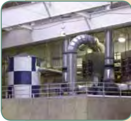
Rainwater collection system
