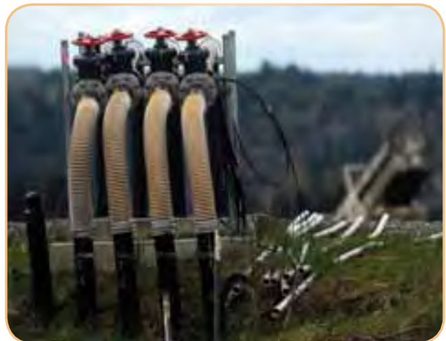
Collecting landfill gas as the garbage decomposes over time is a crucial element of pre- and post-closure maintenance.
