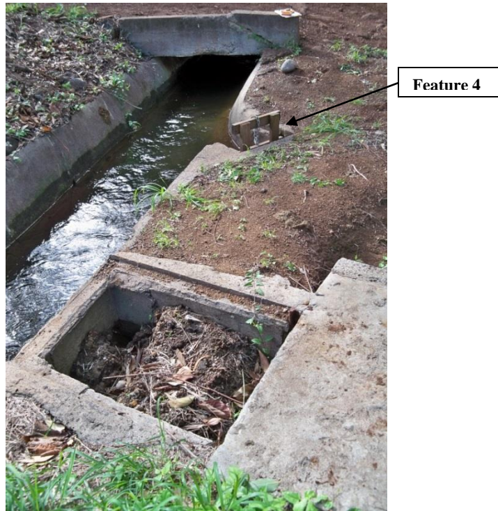
Figure 33. Site 7881 Feature 1 (ditch), Feature 5 (Water Containment Feature) and Feature 4 (Sluice Gate) (View to North)
