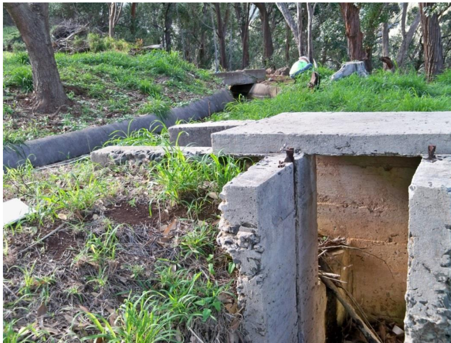
Figure 35. Photograph of Site 7881 Feature 6 foreground with Feature 1 ditch background (View to North)
