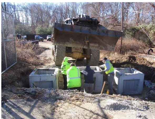
Photo showing the concrete boxes for the sand filters. Credit: Pat Rector
