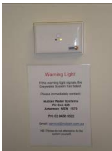
Photo 10: Warning light and procedure at Depot
