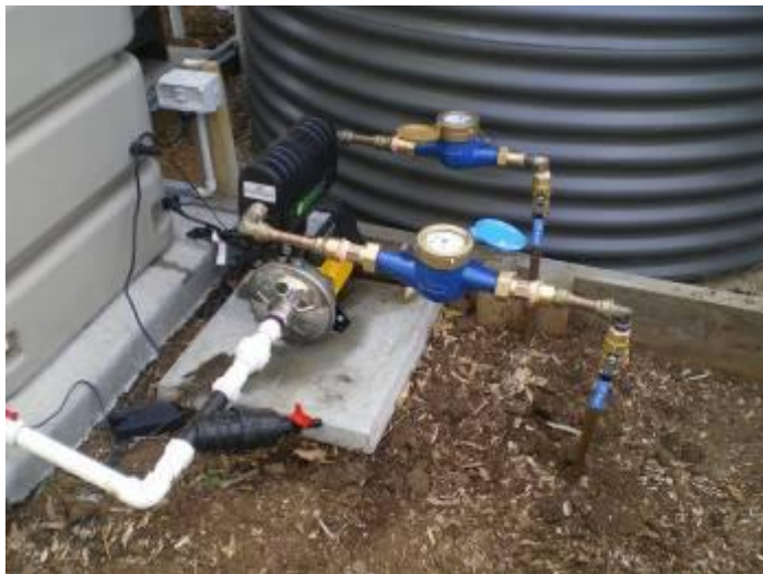
Photo 7: Pipes to the toilet system from the greywater treatment plant and the meters.
