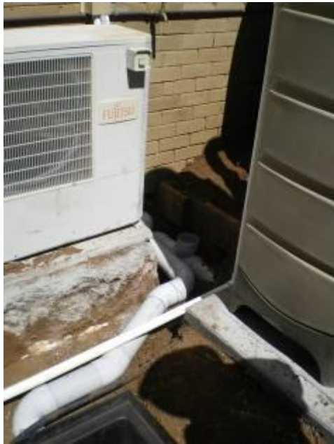
Photo 4: Pipework from toilets to pump well back to greywater system
