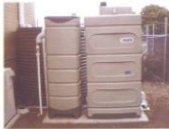
Grey Water System at Warragul Council Depot.
