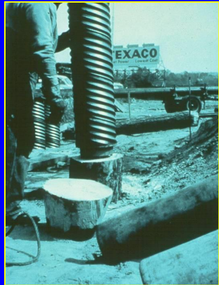
Corrugated Shell - Timber
