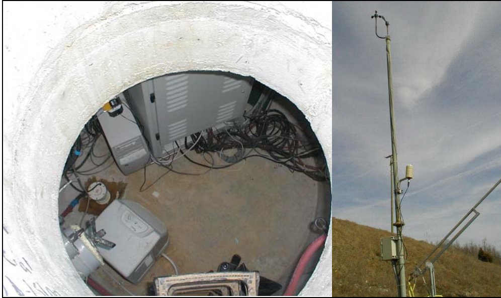
Figure 60. Bunker with DAS and weather station installed on the Smart Road.
