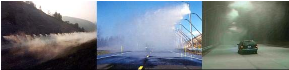
Figure 58. Fog, rain, and snow equipment installed on the Smart Road.
