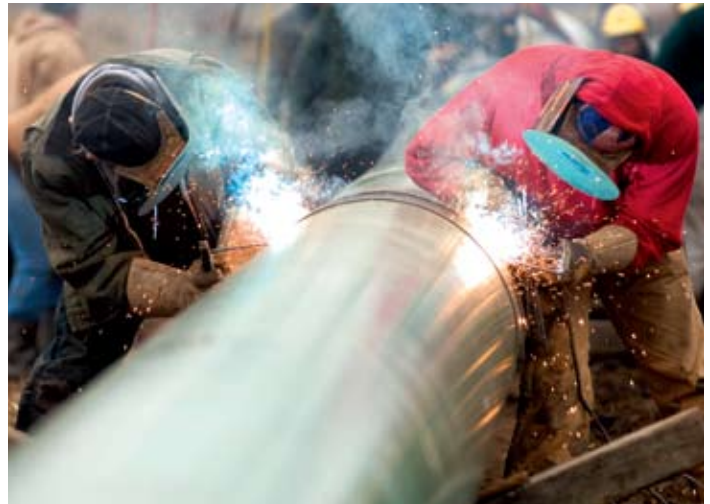
MichCon owns and maintains pipelines throughout Michigan.
