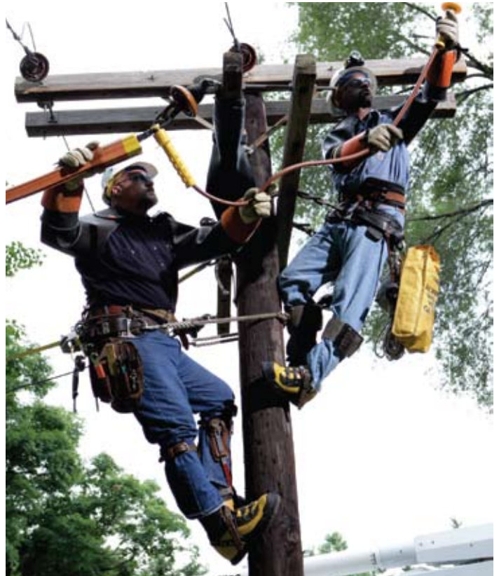
Our commitment to improving customer service includes spending millions to improve the reliability of our electrical system.
