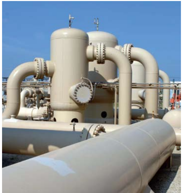
Our Belle River Mills facility is part of a $76 million project designed to capitalize on our storage capabilities and ultimately reduce our customers' exposure to volatile natural gas prices.
