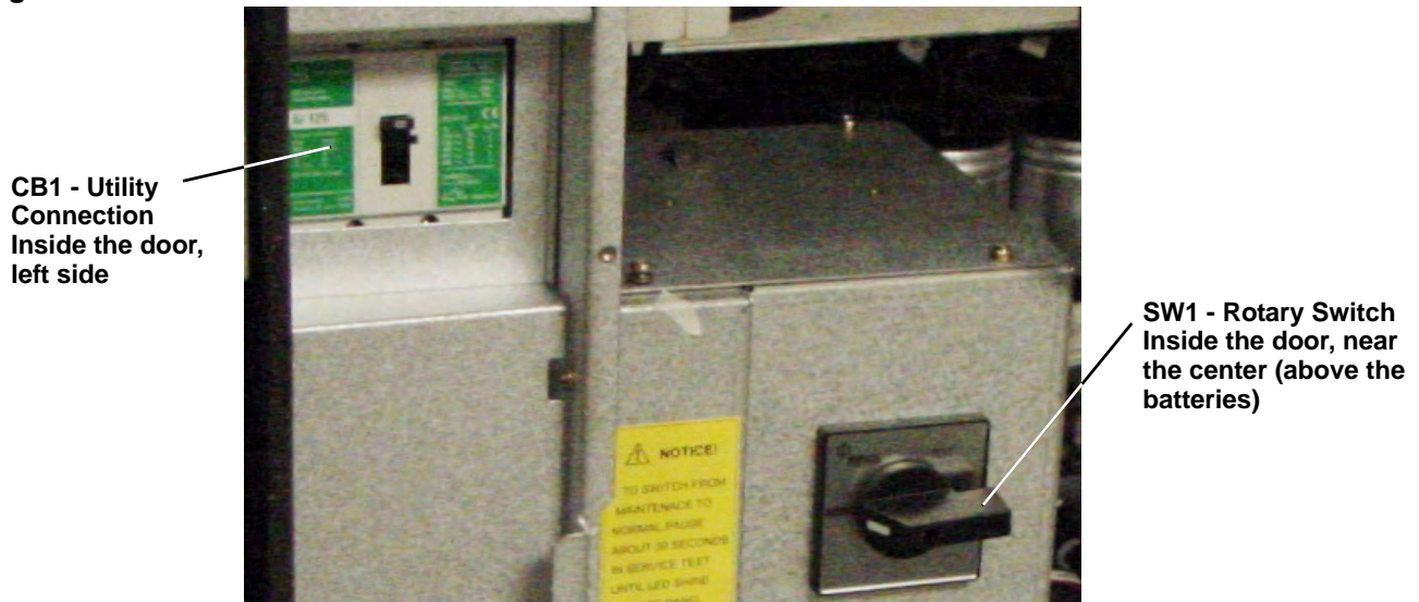
Figure 58 Power switches - 10kVA TRX
