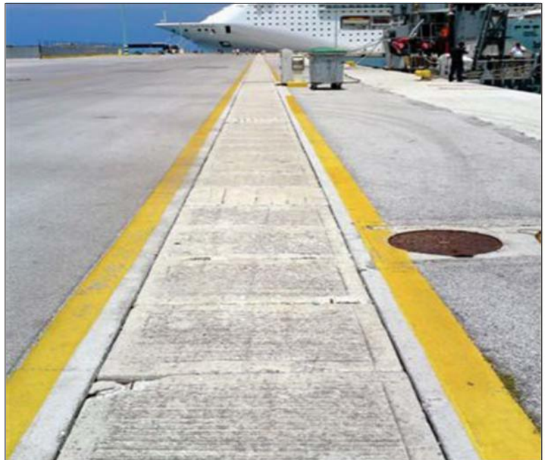
Damaged concrete trench covers in need of replacement to meet Health & Safety Regulations
