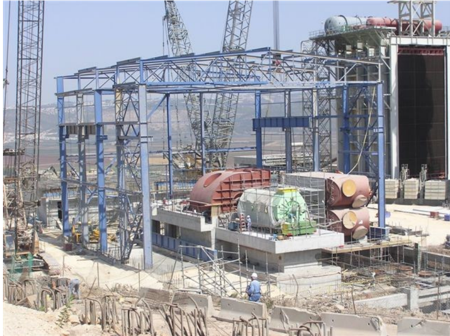
Figure 1: Table-Top Steam Turbine-Generator Foundation
