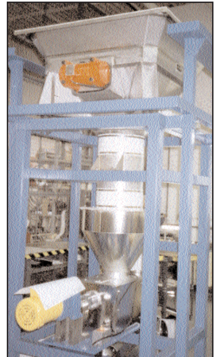
• SCR-100 on Box Dumper to prevent hang-ups
