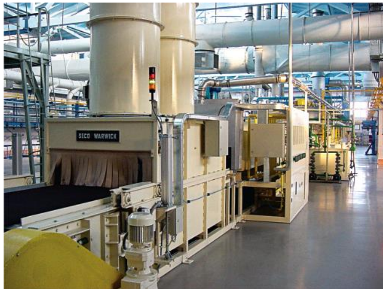
Controlled atmosphere brazing furnace (Source: Seco-Warwick)
