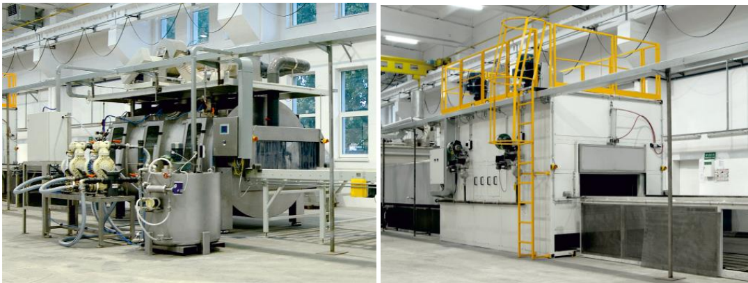
Flux application station (left) and dry off oven (right)
