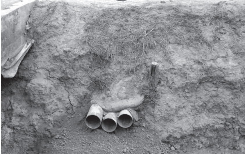
The pipes that carry water from the TC to the rice fields
