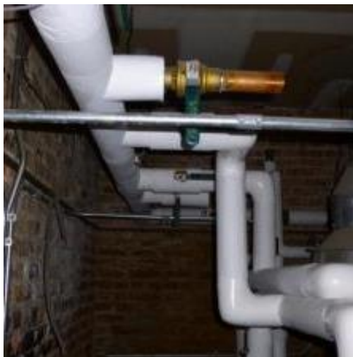
Insulate 100% of hot water pipe
