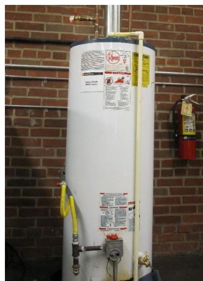
Gas Storage Tank
